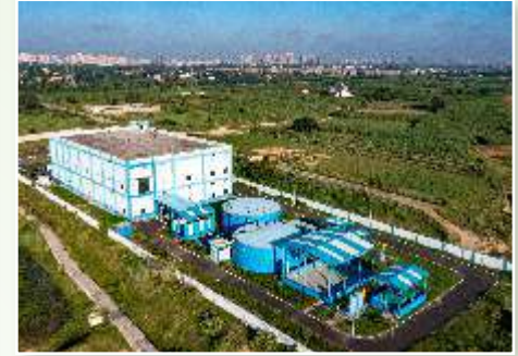
Automated Waste Collection Utility Building and Bio-Methanation Plant for waste to electricity production
