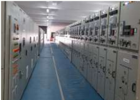
Fully Automated 33/11 Electric Sub-Station
