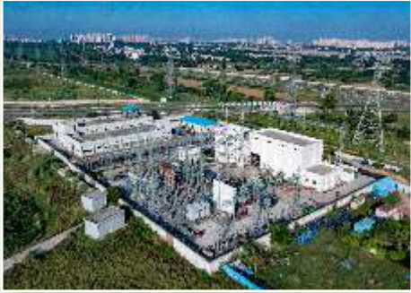
Dedicated 220 KV Power Sub-station supplied by two transmission lines.
